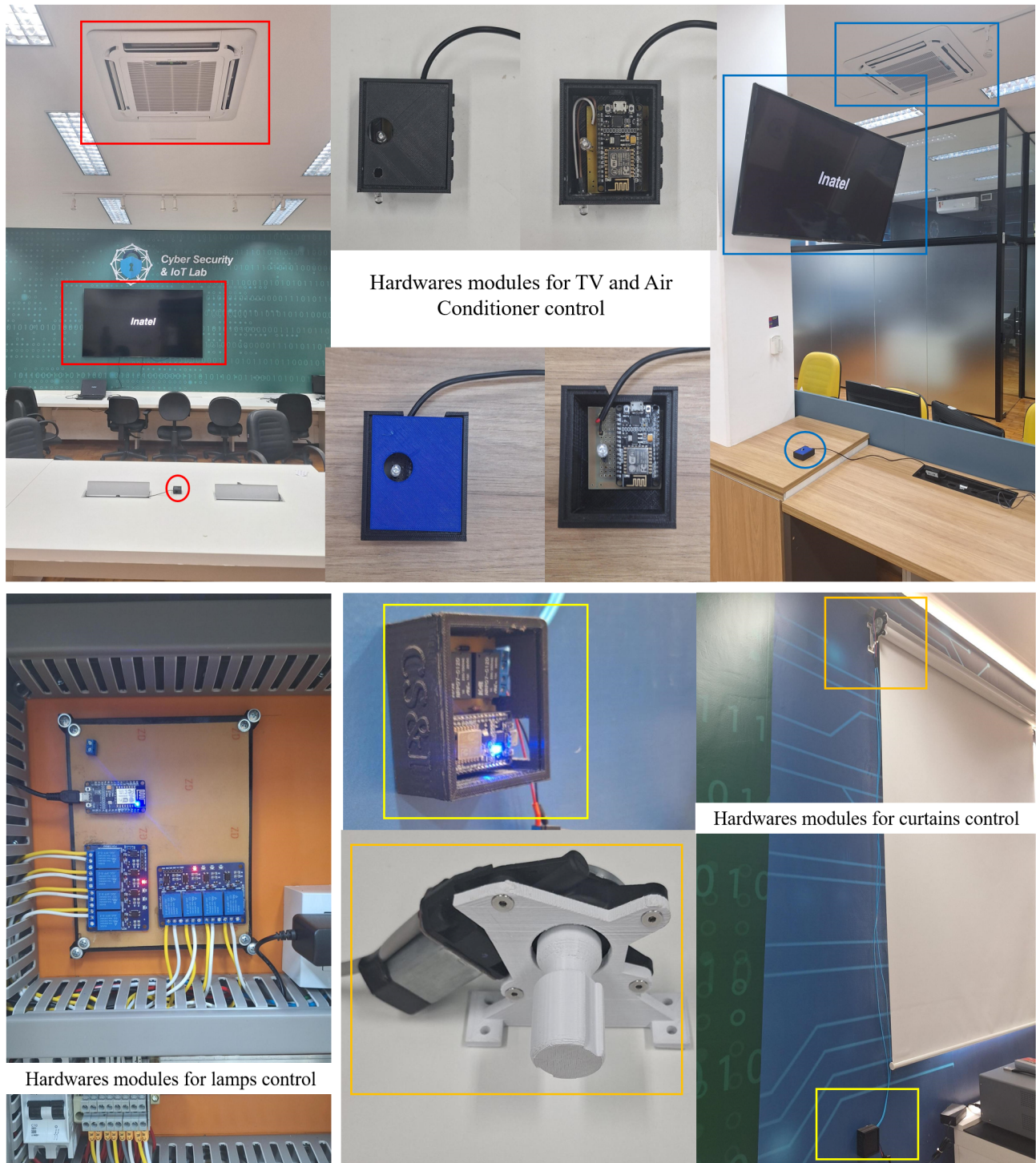
Fig. 5. Hardware modules implementation in the laboratory environment.
